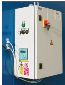
ELECTRIC CONTROL BOARD
